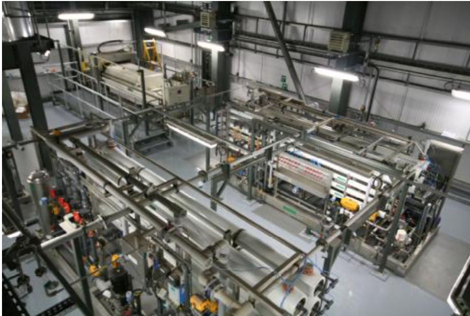
Showing membrane skids and filter press
